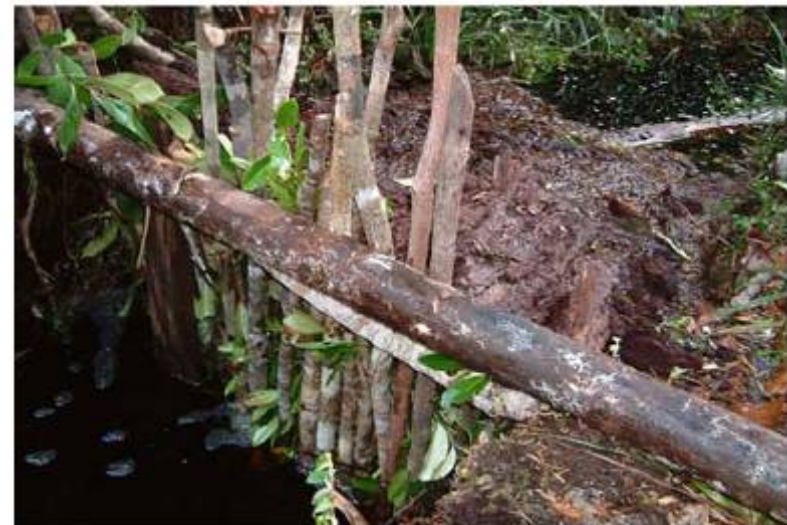
Figure 5. Example of a small dam in an illegal logging canal in the Sebangau peatland constructed using locally available materials.
